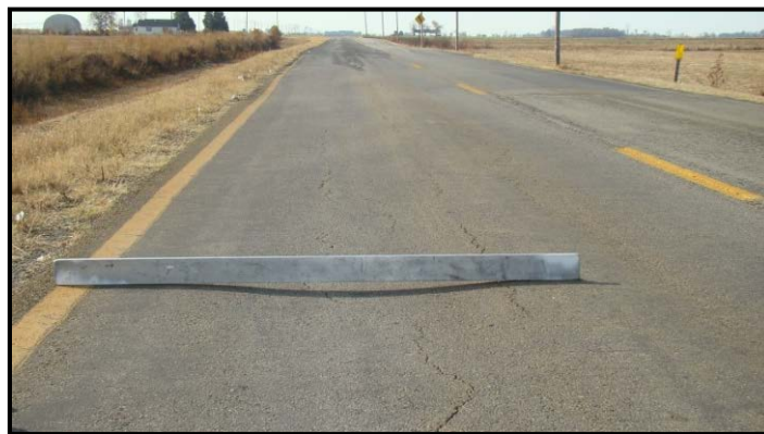
Figure 5: Typical Rutting Found Between Log Mile 8.4-10.46
