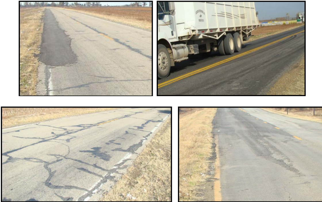
Figure 3: Cracking and Minor Rehabilitation
